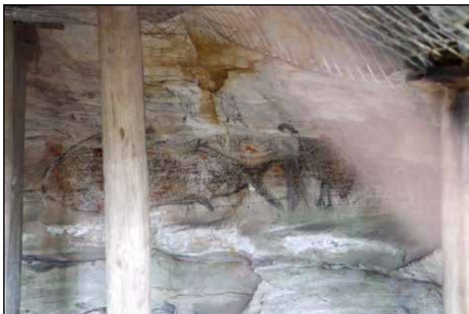
Whale Cave in the Illawarra region has been severely damaged by coal mining activity and the ceiling is held up by timber props. Photo: Tim Fernandez, ABC
