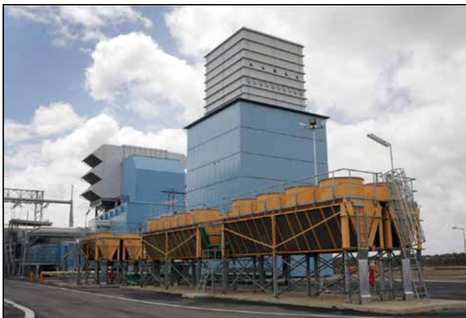
Origin Energy's Mortlake gas-fired power station (pictured in 2012) was damaged in an explosion, with one of its two generators knocked off-line for months. Photo: Rob Gunstone
